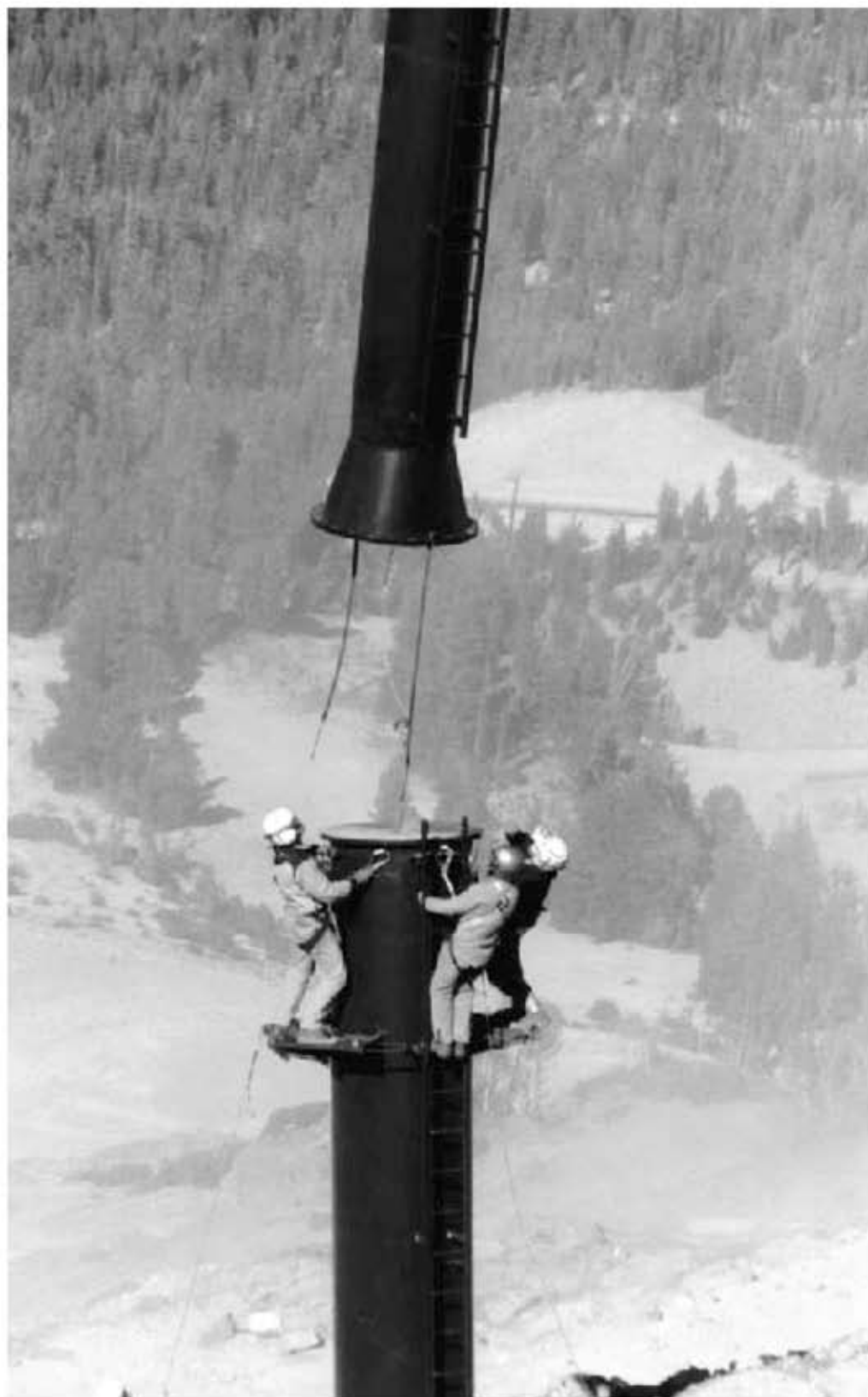
Rusty Gregory, Philippe Mollard, and Heimo Ladinig setting the upper section of the second tower before the top during the rebuilding of Chair 3 in 1997. The helicopter couldn't carry the weight of a full tower, so the crew set the bottom half, filled it with concrete, then added the upper section. Chic Gladding built the circular platform to stand on.
