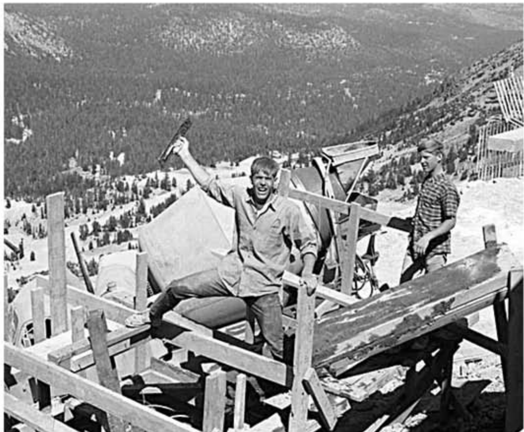
Two days after the accident. Poncho McCoy and David "Tuffy" Mitchell cheering as Dennis Agee arrived with the final truckload of cement for Tower 3.
