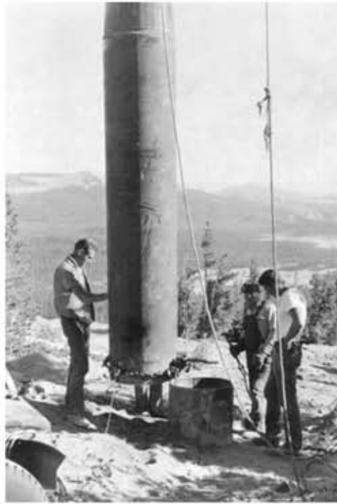
From left: Dave McCoy, Roy the welder, Don Redmon setting a tower.
