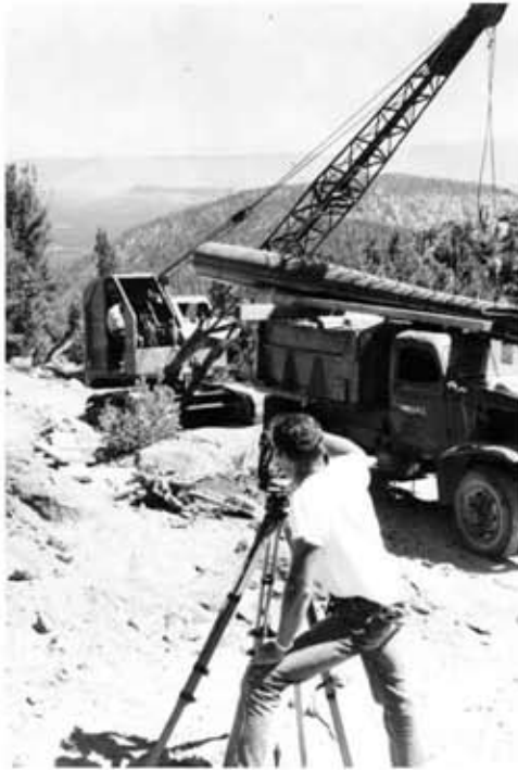
Setting the towers. Don Redmon surveying, Bob Lumkin in crane borrowed from Moffet Lumber.
